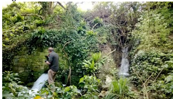
The original outlet on the left of the photo, and the erosion under the road leading to the water ingress on the right
